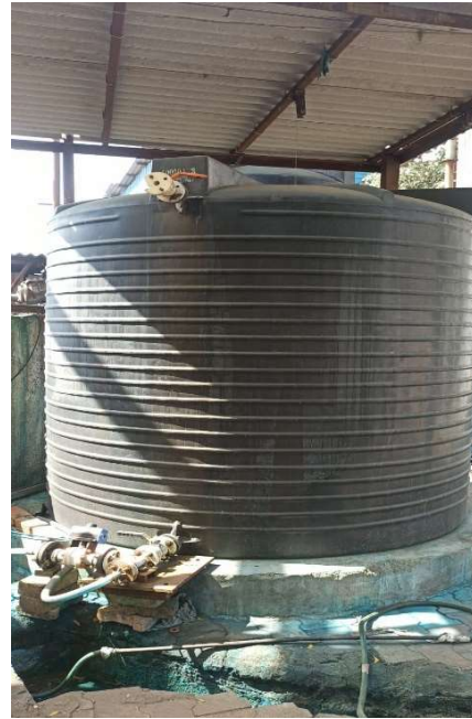
Spent acid storage tank
